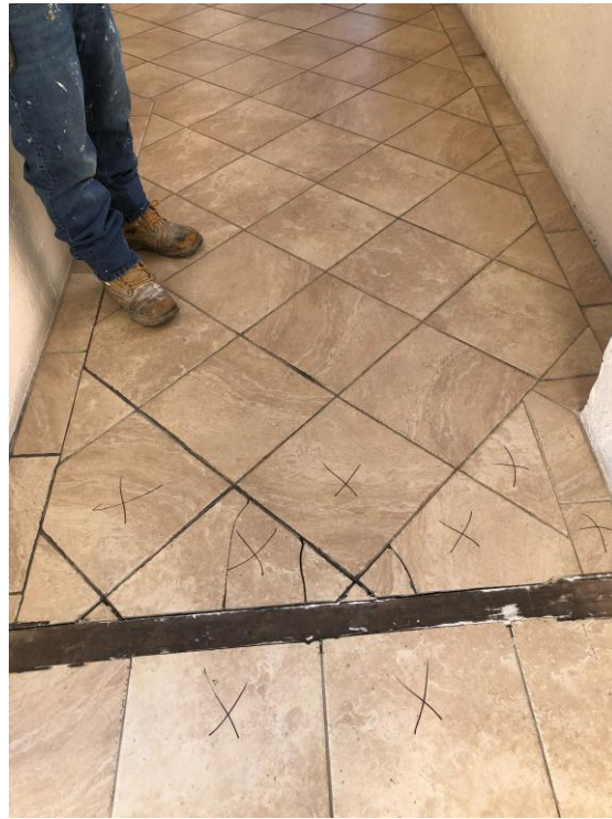
Photo 3: Cracked and delaminated tiles next to the expansion joint
