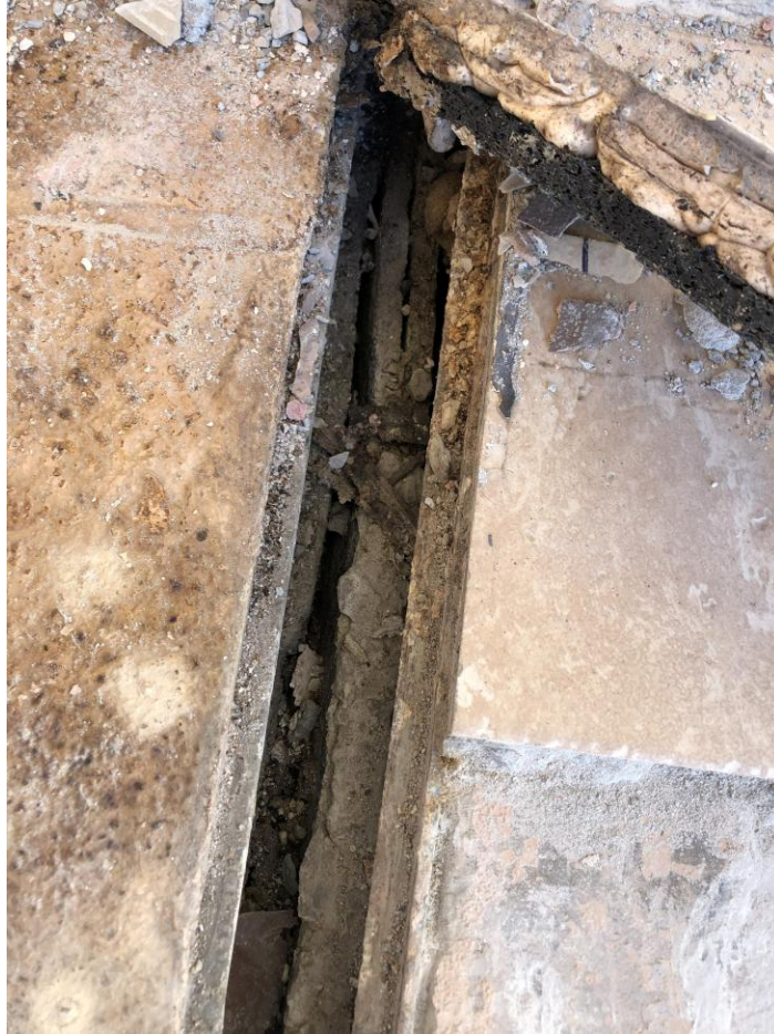
Photo 5: Existing condition of expansion joint after removal of sealant and expansion joint material
