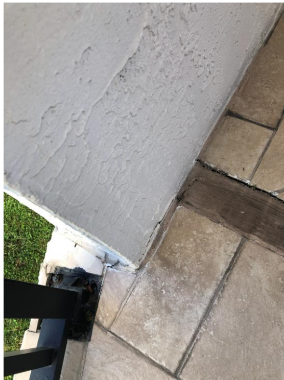
Photo 2: Deteriorated sealant observed on expansion joints
