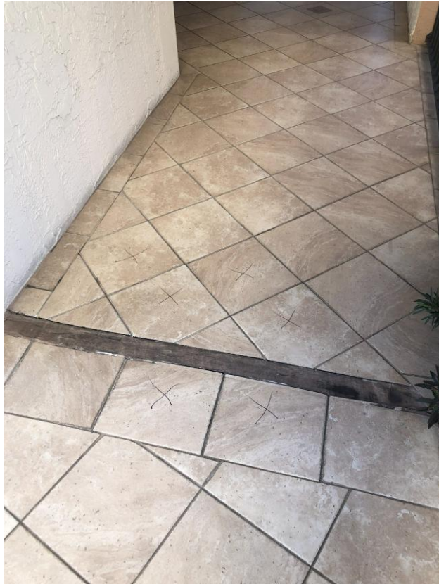
Photo 1: Deteriorated sealant was observed on the expansion joint
